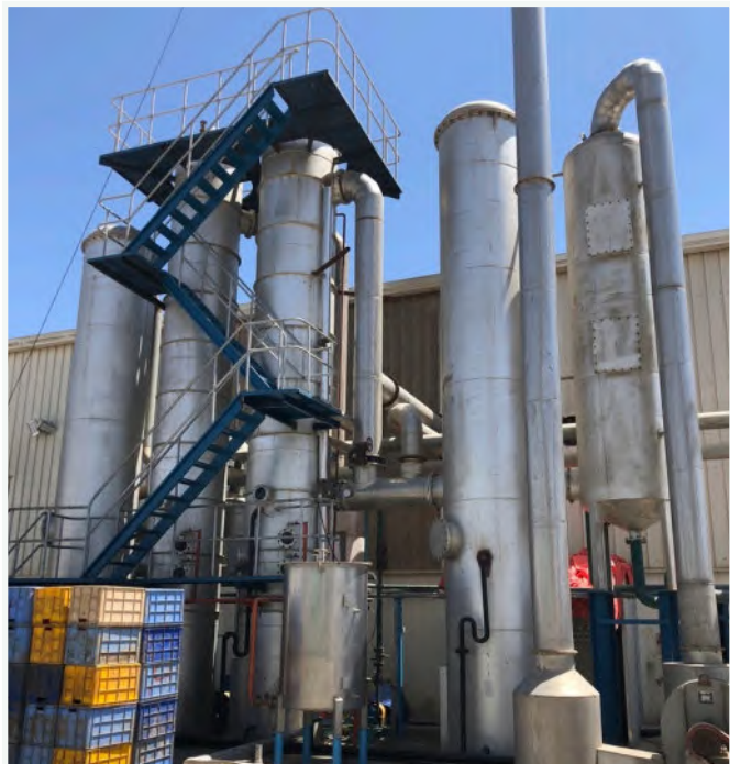
Condenser and washing scrubber
