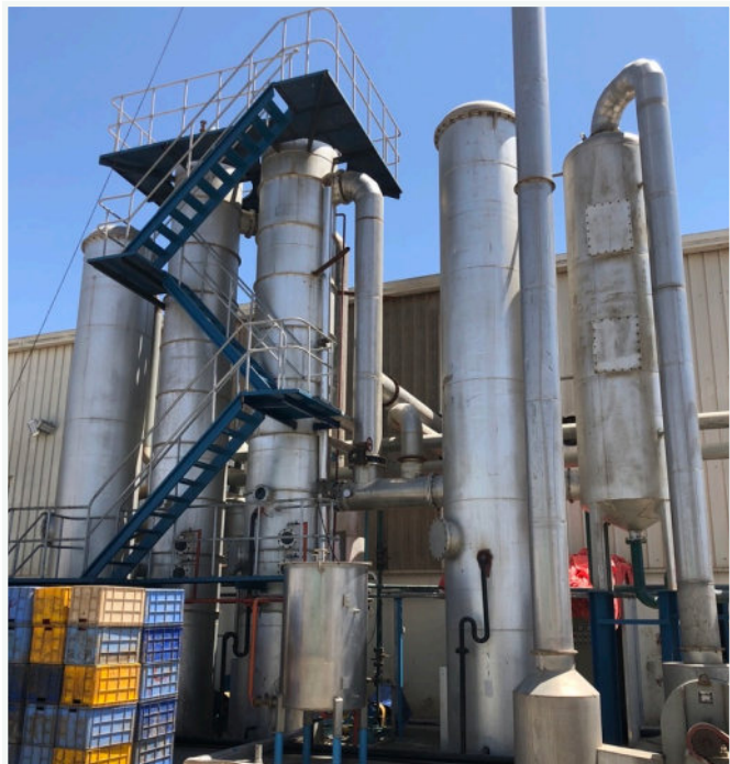
Condenser and washing scrubber
